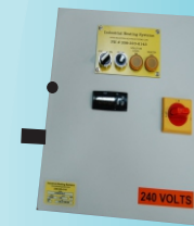
Large Heater Control System
